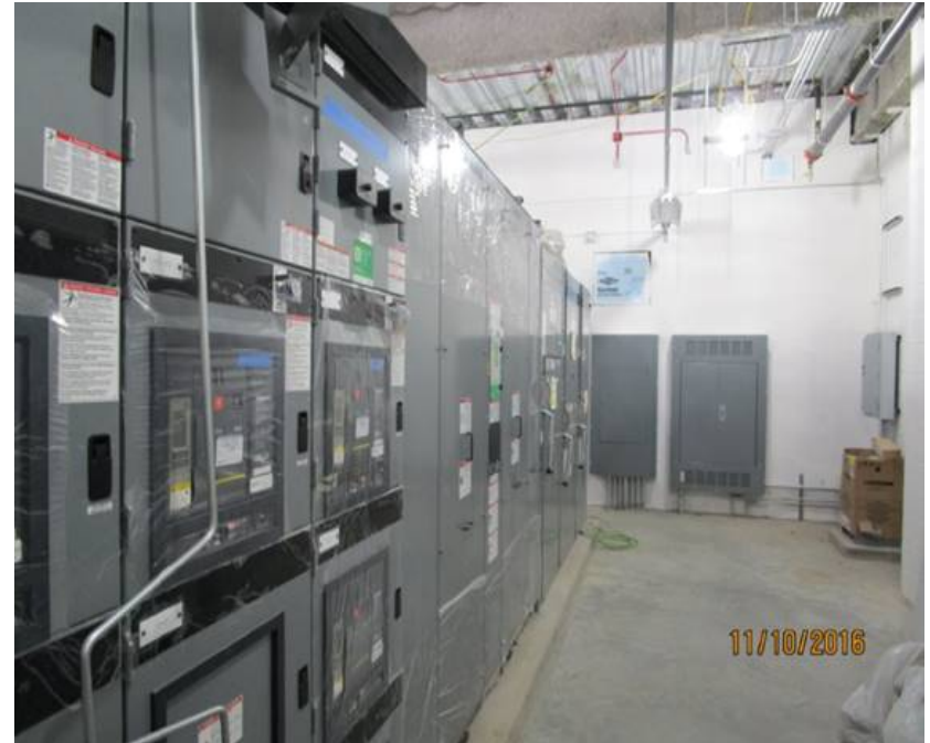
Main electrical gear installed and tied in
