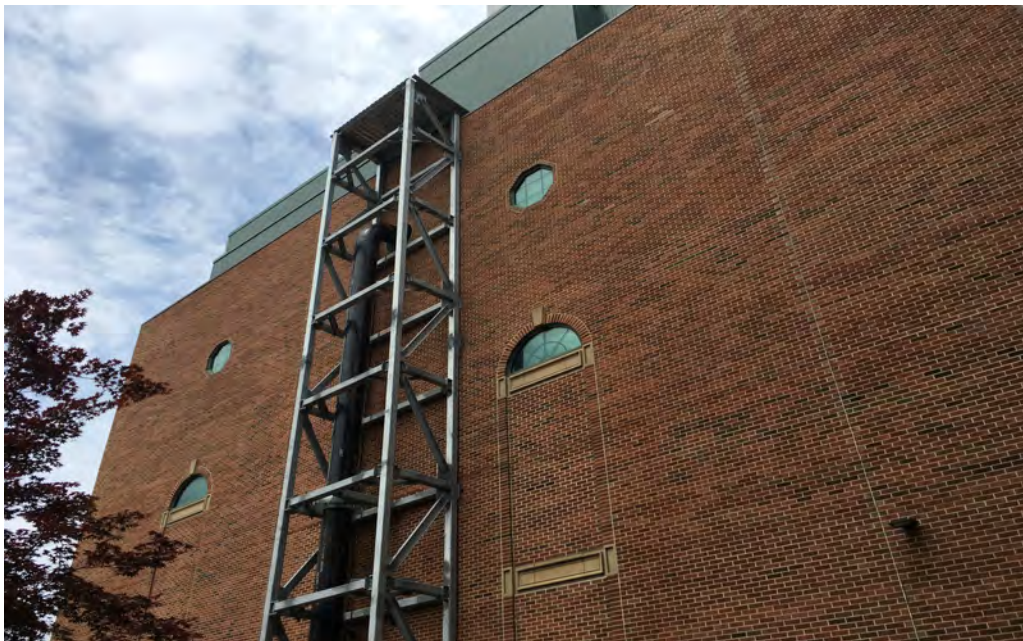
20 inch steam pipe installed in CoGen pipe chase
