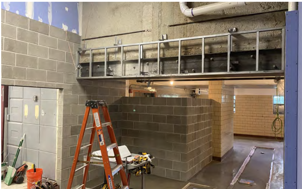
New Accumulator Location
