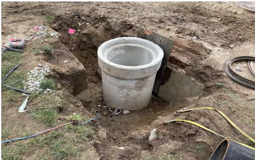
Steam Vault Vent RCP Riser
