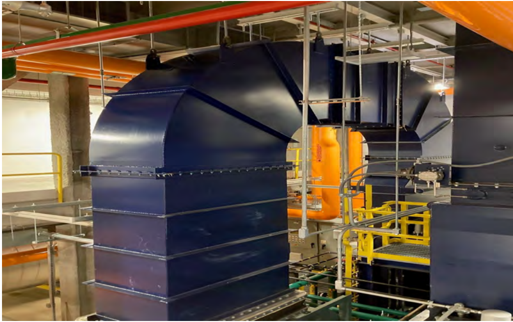
Ductwork painted blue
