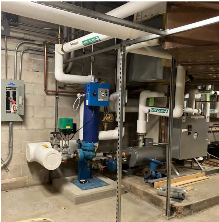
Complete Steam Hot Water Heater
