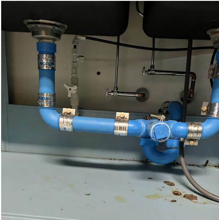
Typical Water Shutoff for Millipore Water Supply
