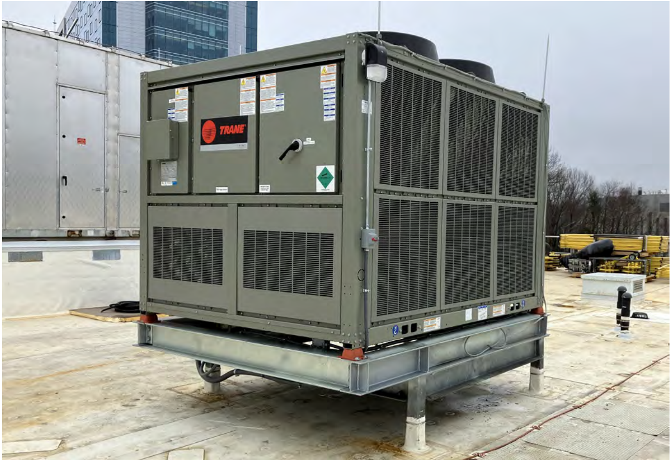
New Roof Top Chiller
