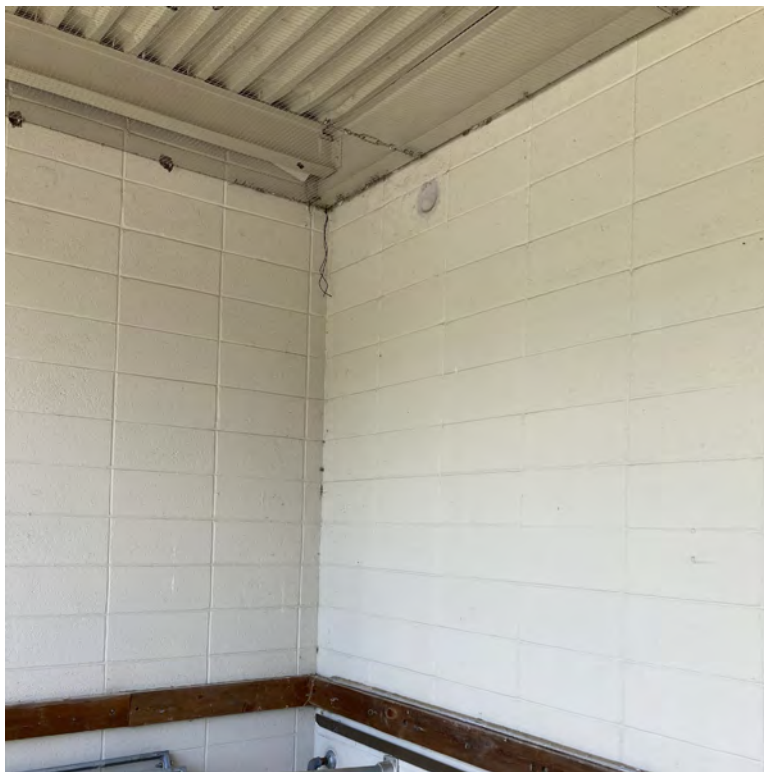
Location of New Ductwork Penetrations into Server Room
