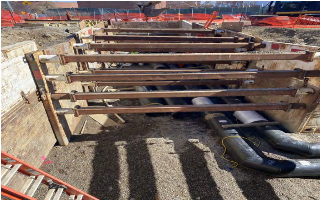
Hot and Cold Water Piping in Lot R (Package 1)
