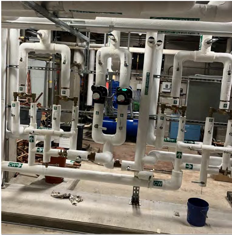
Completed Circulation Pump Station
