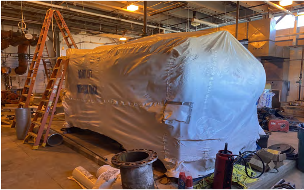
New Gas Driven Chiller in existing Chiller Hall (Package 2)
