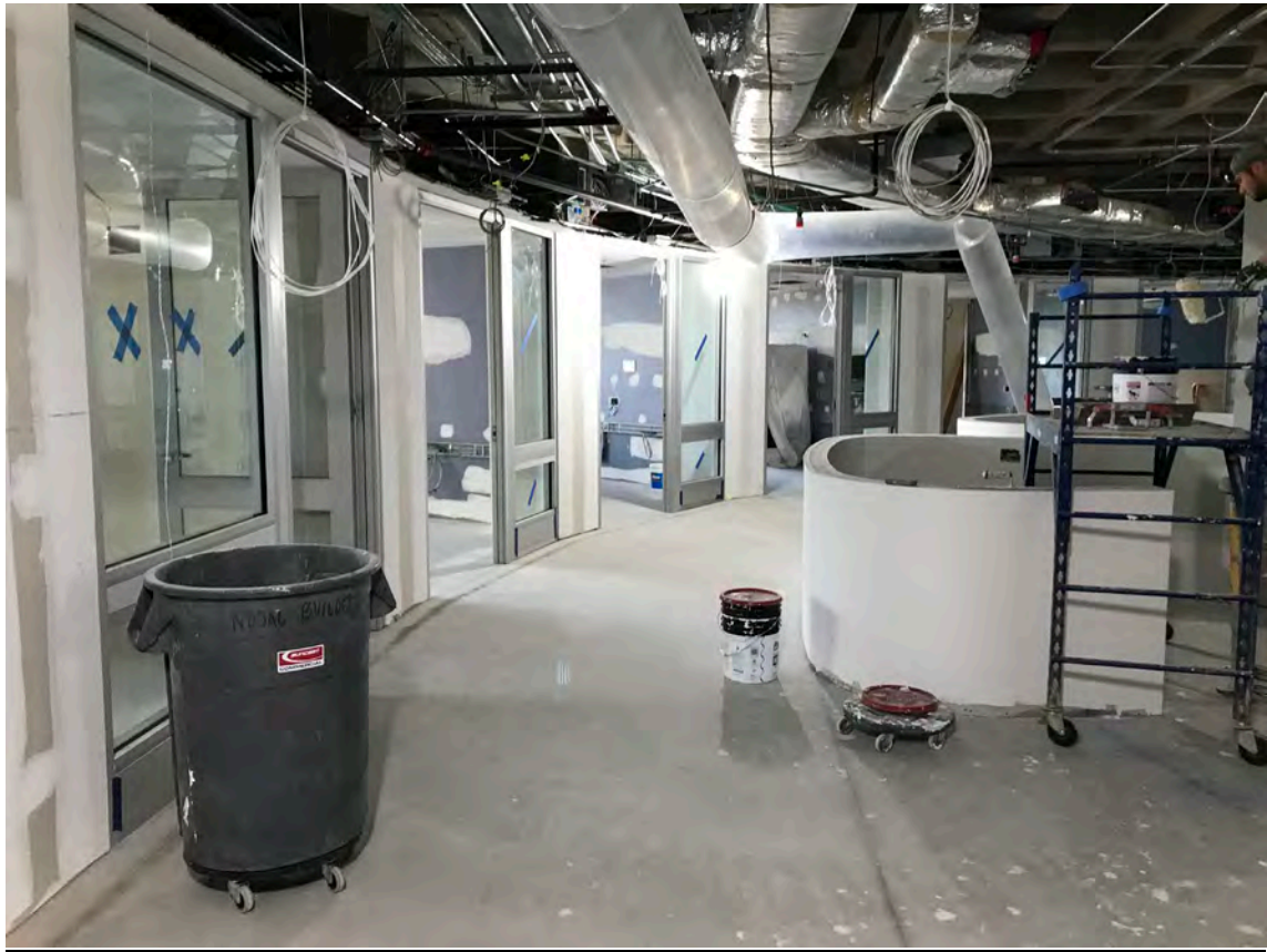
View of Perimeter Patient Room Storefronts & Nurse Station
