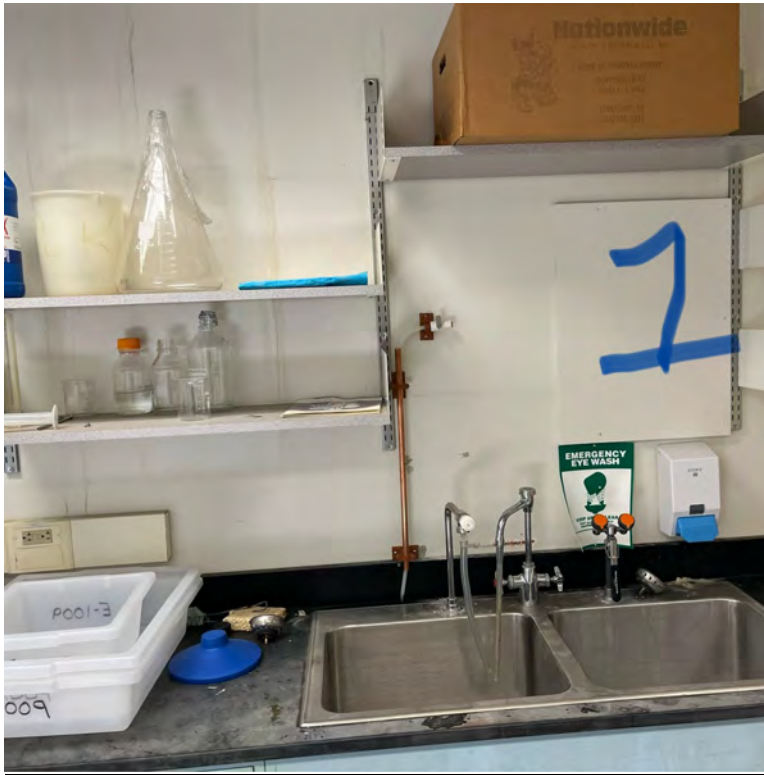
E1009 Millipore Install Location
