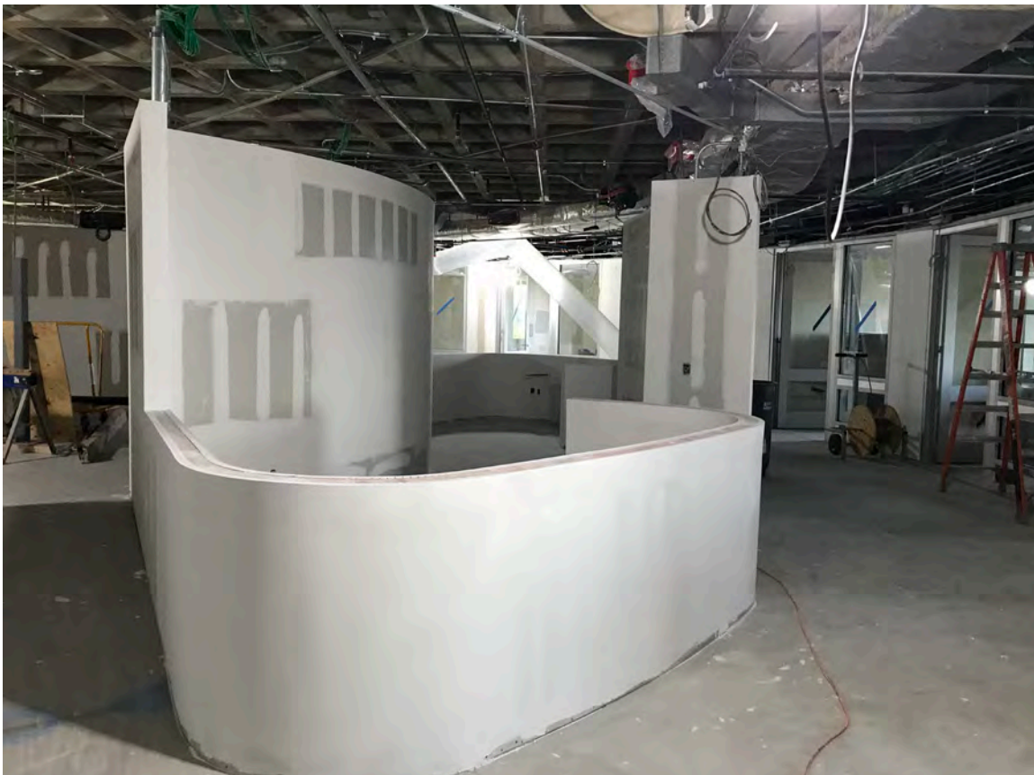
View at New Nurse Station Area
