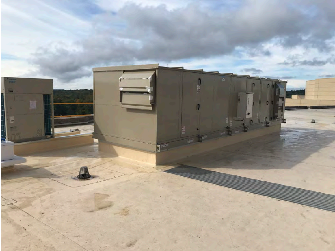
View of new rooftop air handling unit
