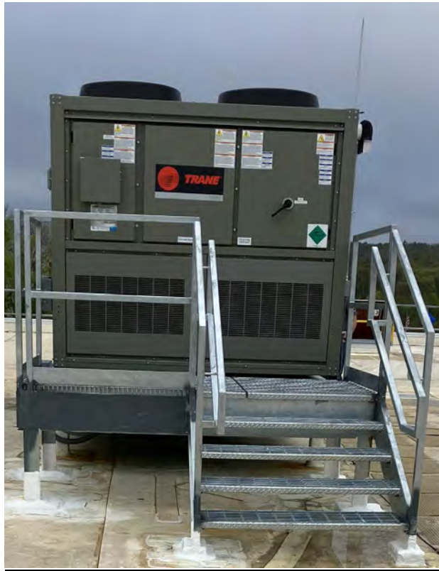
New Roof Top Chiller and Access Stairs
