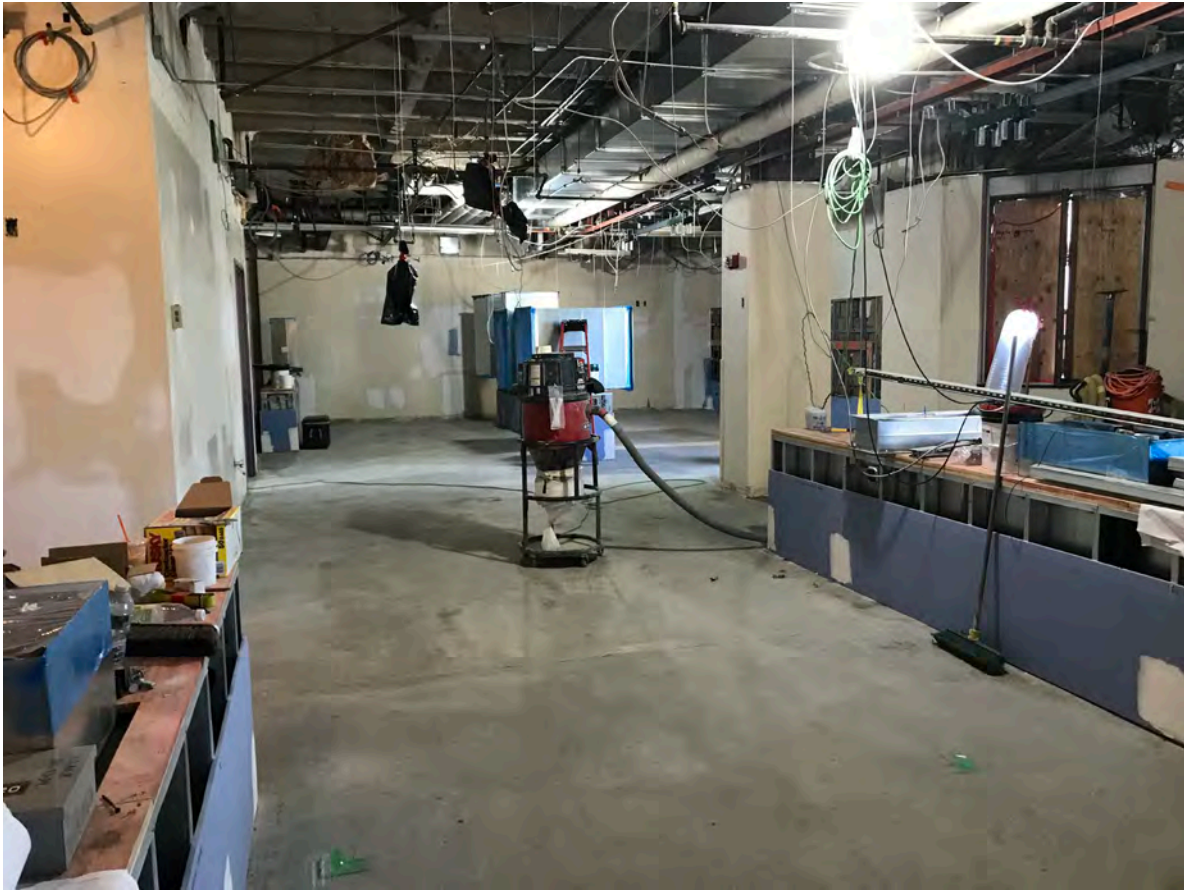
View of Center Portion of Lab
