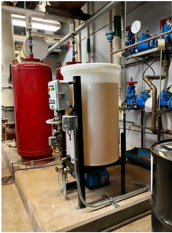
New Glycol System in Boiler Room
