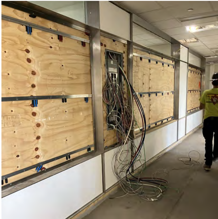
Wiring of Electrical Panel in Main Corridor L2C8
