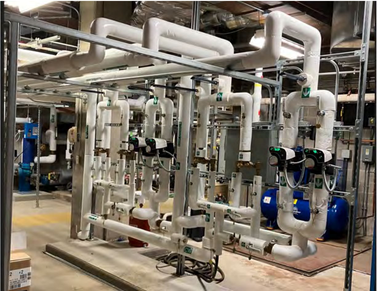
Completed Domestic Water Heating System
