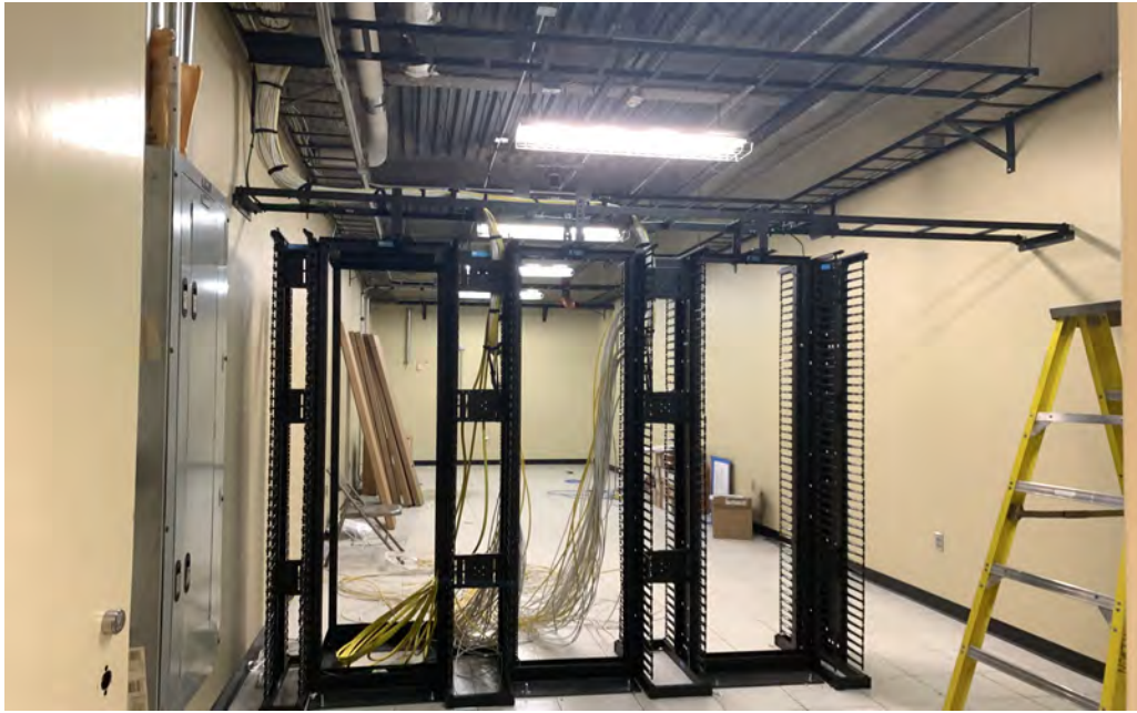
Room 302G Data Closet - new equipment racks installed
