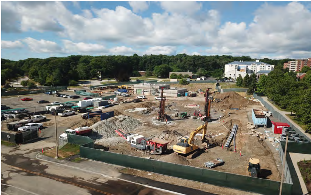
Geothermal Field Looking SW (Package 2)
