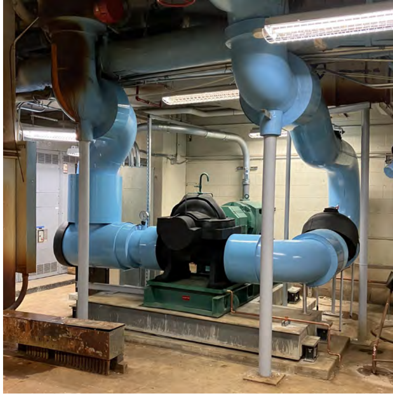
Chilled Water Pump #4
